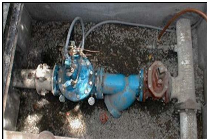
Gambar2.7 Instalasi Pressure Reducing Valve
