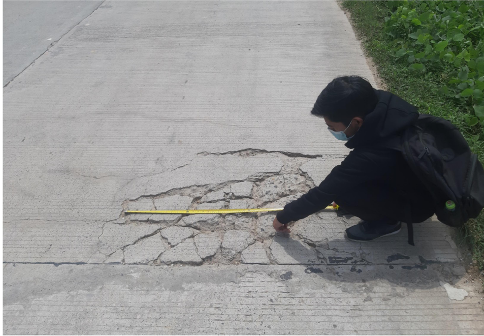
Kerusakan Gompal Sudut ( Spalling Corner )
