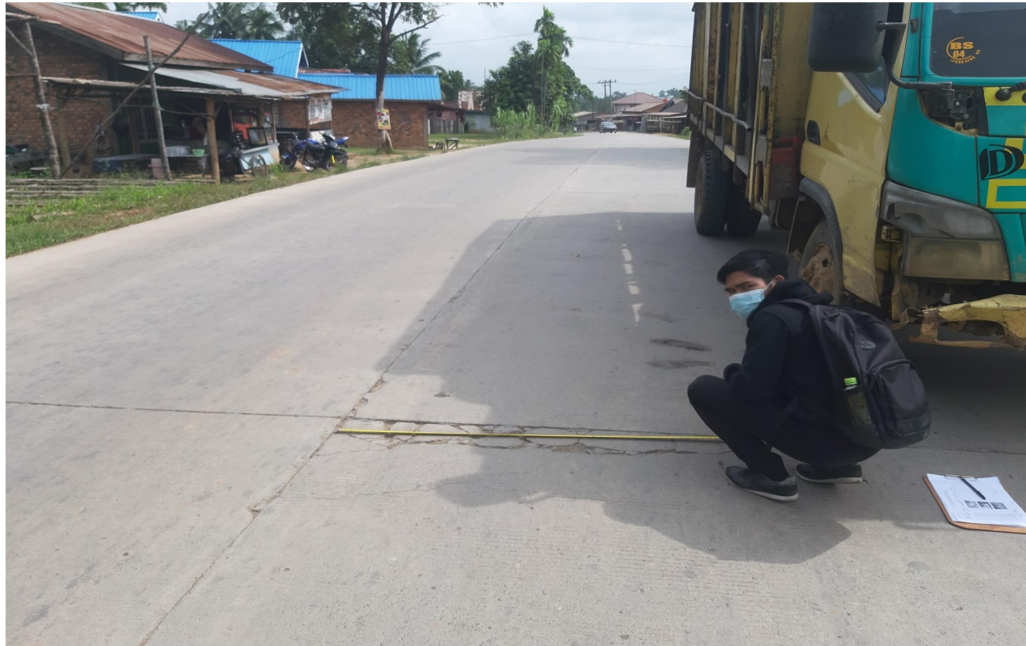
Kerusakan Gompal Sambungan ( Spalling Joint )
