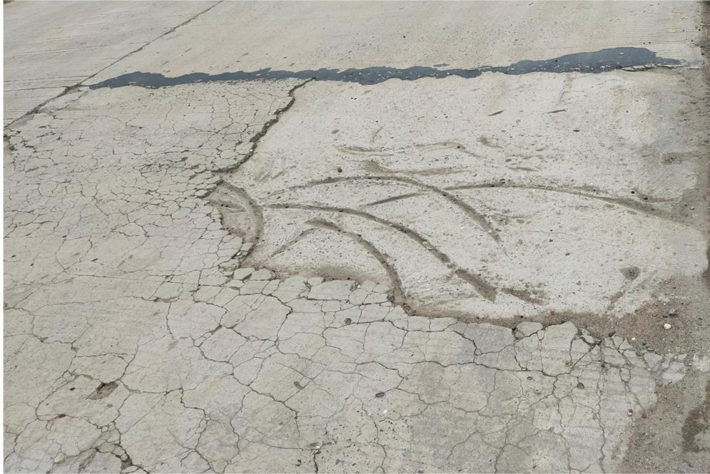
Jenis Kerusakan Gompal Sambungan ( Spalling Joint )
