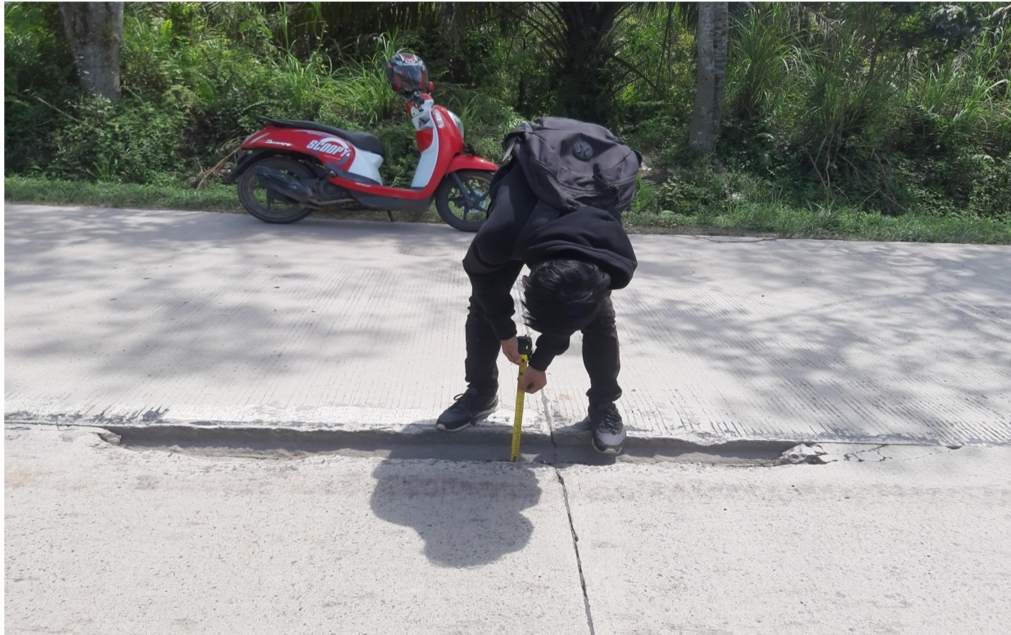
Penutup Sambungan ( Joint Seal Damage )
