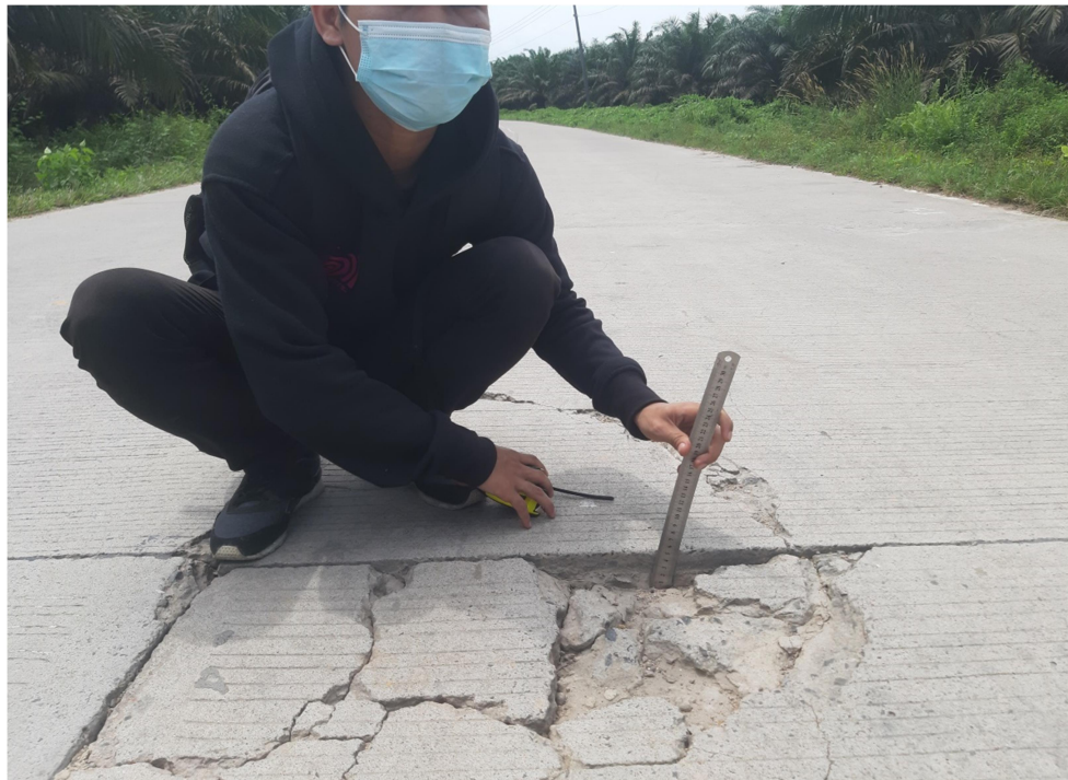
Kerusakan Gompal Sudut ( Spalling Corner )
