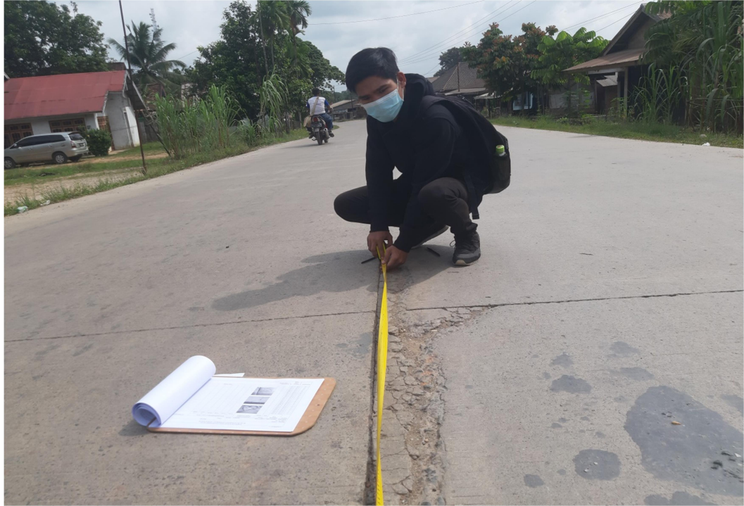
Kerusakan Gompal Sambungan ( Spalling Joint )
