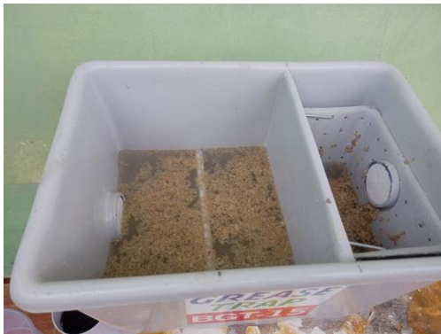
Gambar.11 Kondisi Air Limbah Didalam Grease Trap
