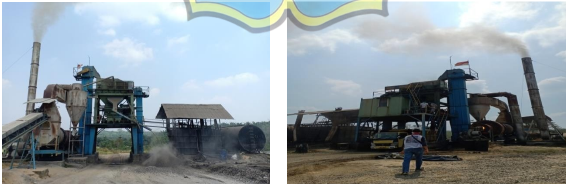
Asphalt Mixing Plant
